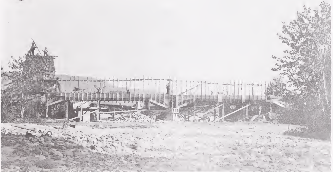
This photograph shows the bridge with frame for the concrete forms still in place. The mixing plant is on the left. The bridge was structurally similar to the Conley Street Bridge in Deer Lodge (Montana Historical Society).
